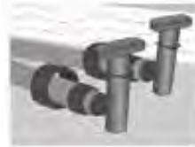
Low Point Drains
