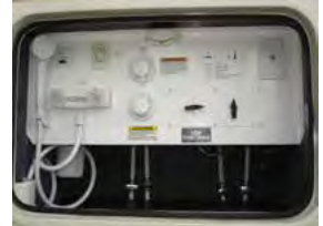
Fig. B - Utility Center
