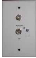
Antenna Power Supply
