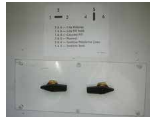
Fig. A -Water Valve Controls
